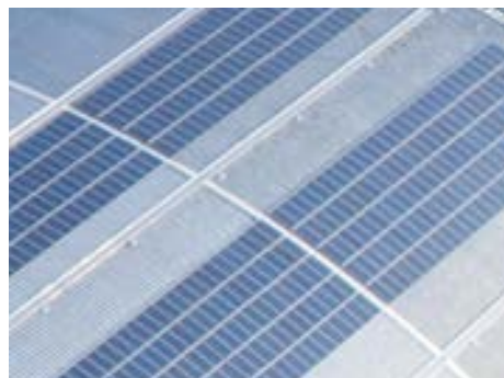
Solar panels installed on the roof of the terminal.
