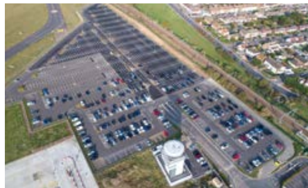
The expanded long stay 3 car park which was completed by Stobart Rail & Civils.
